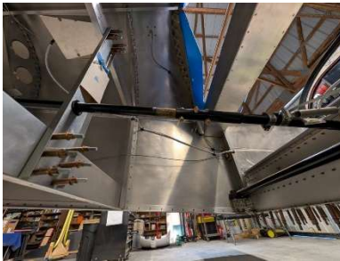
ADHRS cable routed
