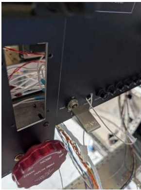
Flap switch installed in panel
