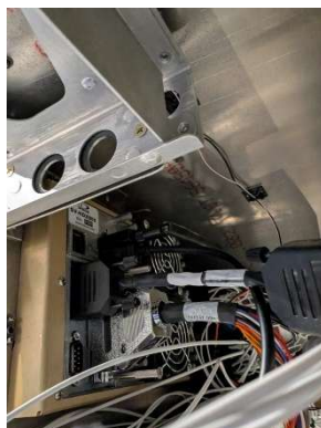
SkyView USB extension and Wi-Fi adapter installed
