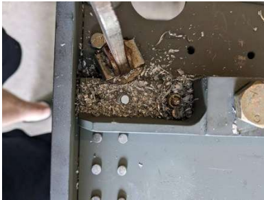
Enlarged rigging block hole
