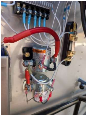
Master relay control and diode added
