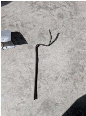
Hard fuel vent line cut and bent
