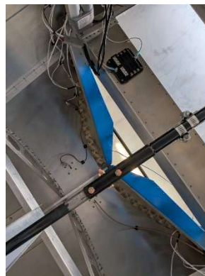
Ground and power feeds ran to aux fuse box
