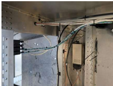
AP servo wiring connected to SV-NET-HUB under crosstie
