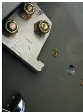
Oversized bolt installed
