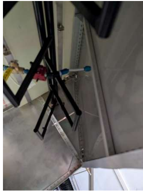
Hardline installed between tank and bulkhead fitting
