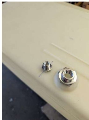
Fuel sender fitting installed
