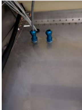
Cable bulkheads installed
