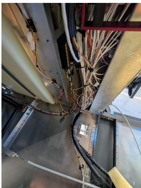
Panel wiring secured
