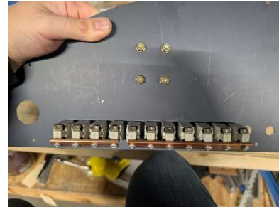
Circuit breakers and bus bars installed
