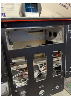
Garmin GPS175 tray installed
