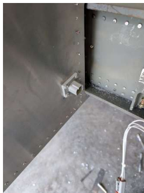
LH bulkhead connector installed
