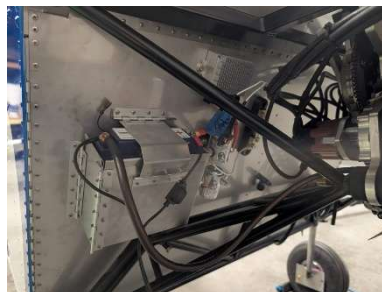
Electrical distribution cables made
