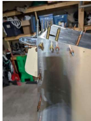
AN525 holes drilled through aft fuselage floor and lower splice plate
