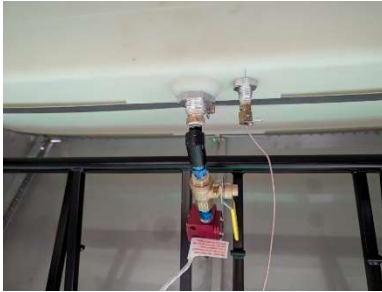
Fuel probe installed
