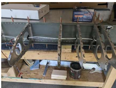
RH inboard wiring run
