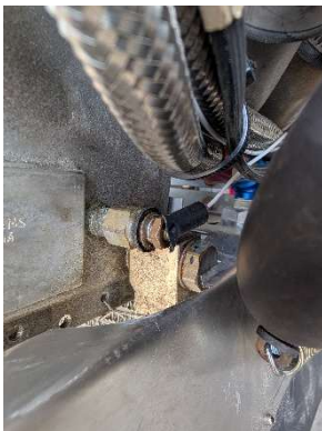
Oil temp probe protected
