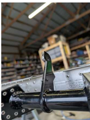
Small amount of material removed from elevator horn
