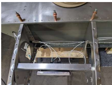
RH landing light wiring with maintenance loops
