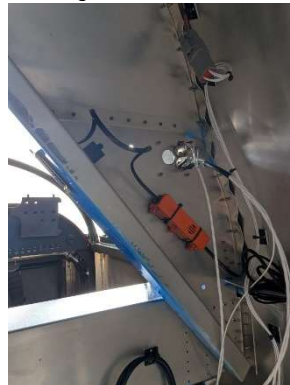
Audio alert module mounted and wiring connected
