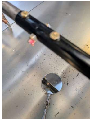
Torque seal added to elevator pushrod bolts
