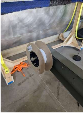
Setup for easier wiring runs
