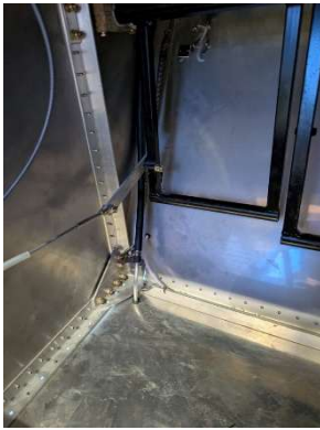
New fuel vent line connected to fuel tank breather
