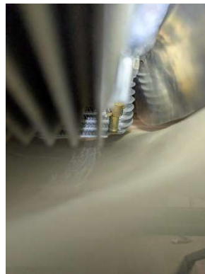
Oil cooler interference
