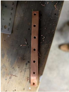
Main bus bar cut and drilled
