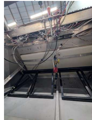
Control cable routing
