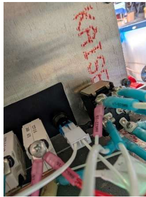
Flap and alternator reset switch wiring behind panel
