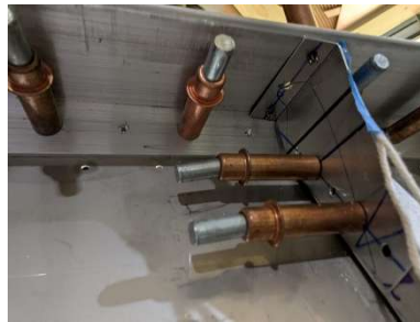
Firewall angle updrilled
