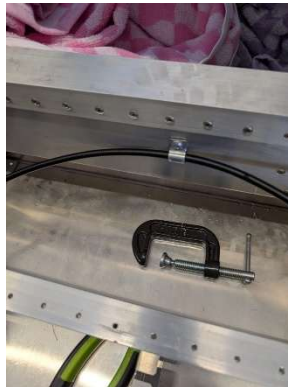
Trim cable secured to rear spar carry through
