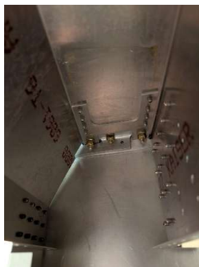
RH former bolts inside cross-tie box
