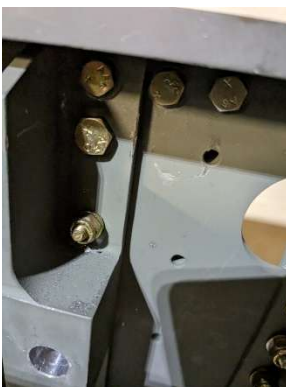
Oversized bolt installed
