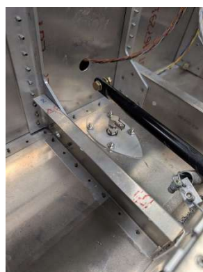
Com antenna installed
