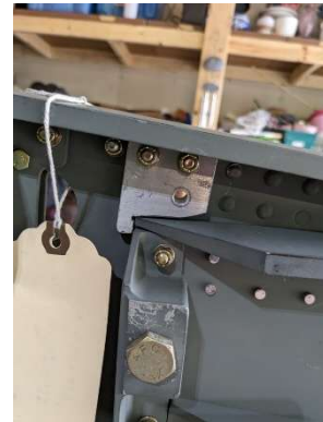
Rig plate missing oversized bolt
