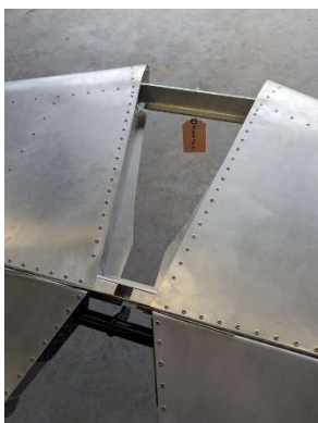
Stabilizer skin installed upside down
