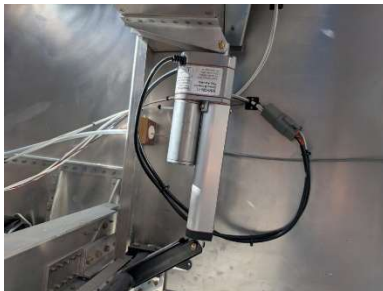
Flap motor wiring
