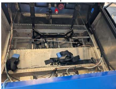
Under seat wiring bundles secured
